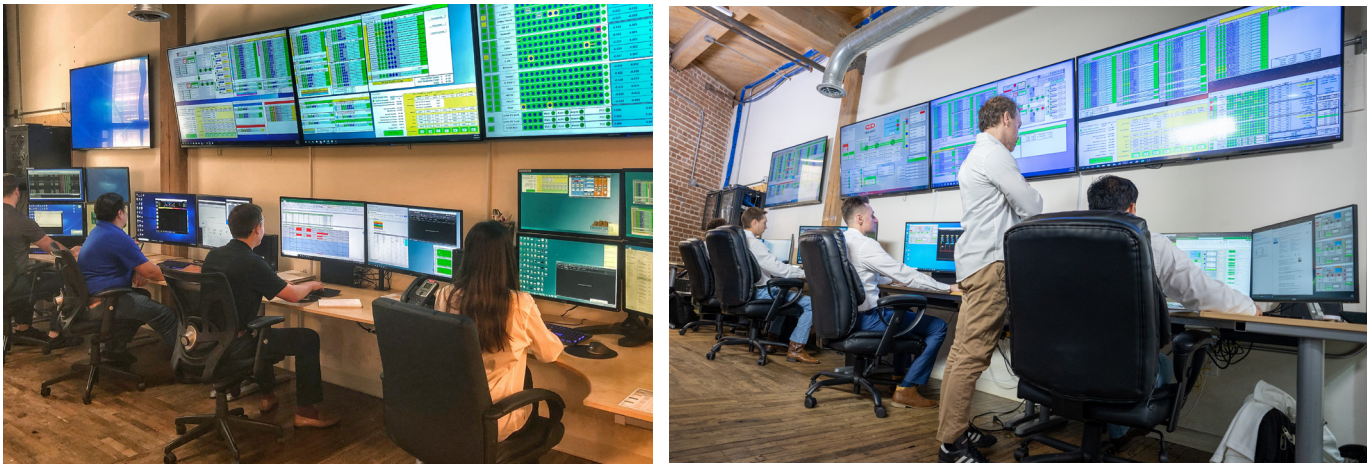
Microgrid Network Operations Center in Houston, TX
